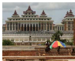
The new parliament building under construction in Naypyitaw: September 2010. Photo: The Irrawaddy online Journal .
